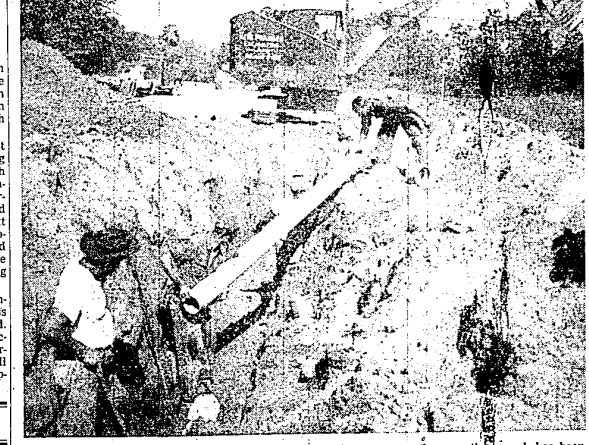
THE INITIAL PHASE of the expansion and improvement of the City Water System was begun late last week with the installation of a new main along the Farmington Cut-Off. The line will extend from the new wells, south of the Cut-Off and west of Farmington Road, to a connection with the existing system on Grand River near Pickett. In the meantime, work has been started on the installation of piping equipment at the well sites. Officials estimate that the project will be completed in approximately two weeks. The additional supply of water is expected to result in a lifting of the present sprinkling restrictions.
