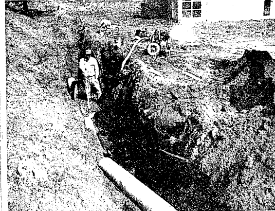
INSTALLATION of shut-off valves on water mains from the new wells to the existing city water system was hampered last week by heavy rains. A workman can be seen above pumping rain water from a section of the excavation. Removal of the water was necessary before the shut-off valves or hydrants could be installed. Some sections of water main must still be placed before the tie-in can be completed. While work on the laying of mains continues, pumps are being transferred and preparations are being made for construction of pump houses at the new well site.
