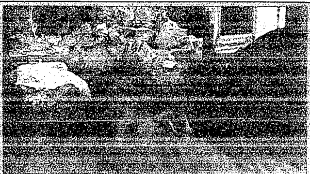
Tom Noble marks each stone with a number — the historic bricks in its original form at the 12 before removing it from the Harger House, Hills Road location. The code numbers will be used to reassemble.
