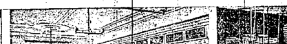
7. Following telegraph methods, connections on this "plug-board" switchboard were made by inserting solid metal plugs between horizontal cross-connecting bars and vertical rows of metal buttons connected to the various lines. Figure 8: The most striking change, as exemplified in today's manual switchboard, is the great compression of equipment required to handle the concentrated traffic of the present.
